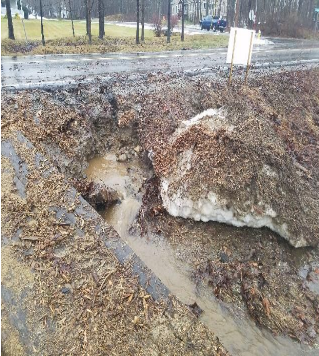
Fig 5: Bank eroded away off of Nimble Hill Rd, flooding Frink farm. Viewing east. (12-14-19).
