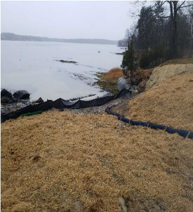
Fig 11: Restoration of slope at Getchell property/west side of the Bay. Viewing east. (12-14-19).
