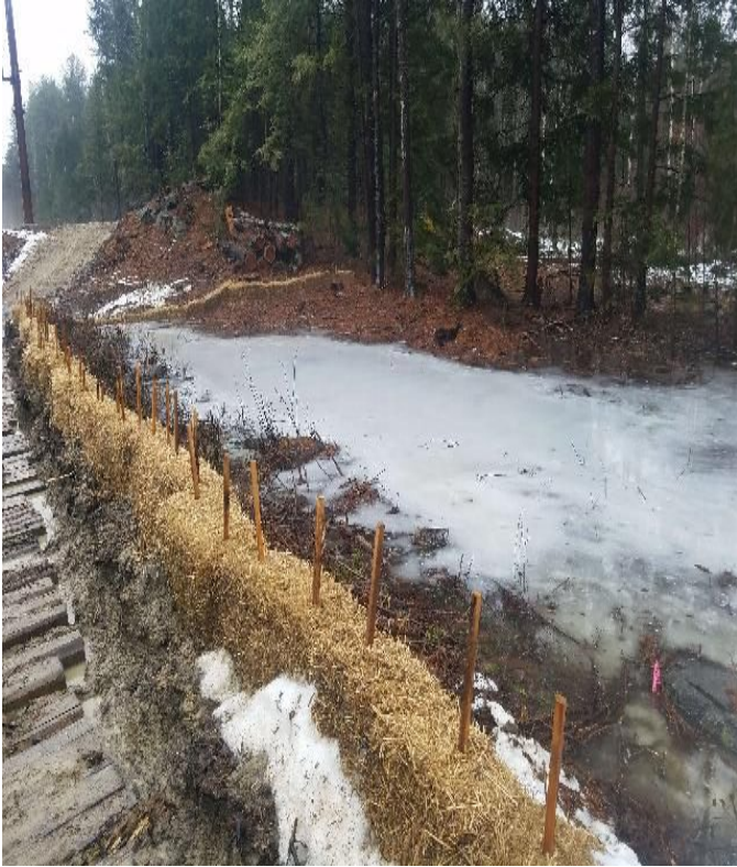
Fig 17: Wetland DW400N iced over, no issues. Viewing south. (12-14-19).
