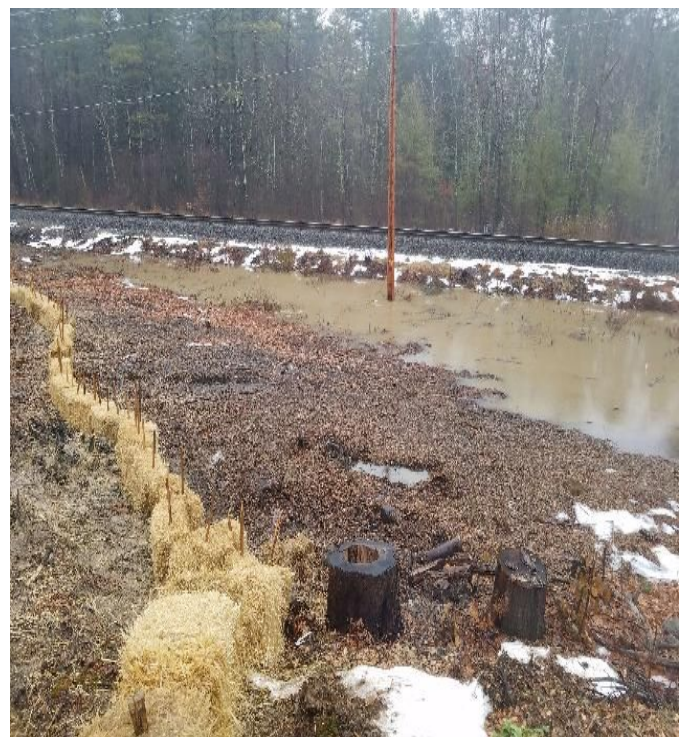
Fig 20: Sediment discharging into wetland MW1 between Strs. 5 and 6. Viewing south. (12-14-19).
