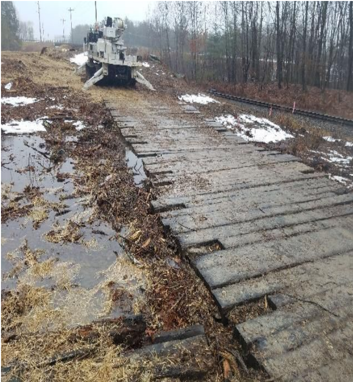
Fig 25: No required BMPs installed along access road through wetland DW93. Viewing south. (12-14-19).
