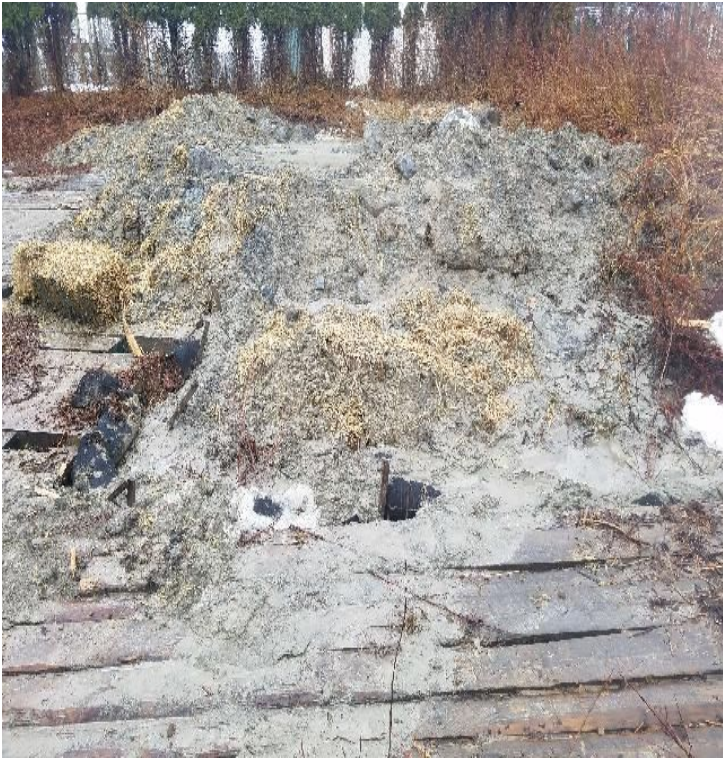
Fig 21: Soil pile at Str 1. Sediment overtopping filter sock. Viewing east. (12-14-19).
