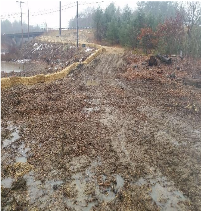
Fig 19: Ruts and exposed soils in access road to Strs. 5 and 6. Viewing south. (12-14-19).
