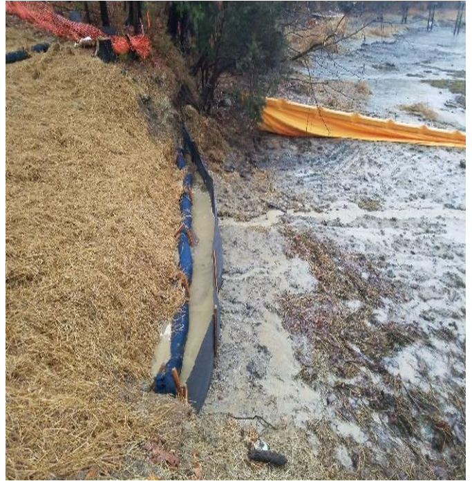
Fig 2: Sediment build up at silt fence. Note undercutting. Turbid water mostly contained by turbidity barrier. Gundalow Landing. Viewing south. (12-14-19).
