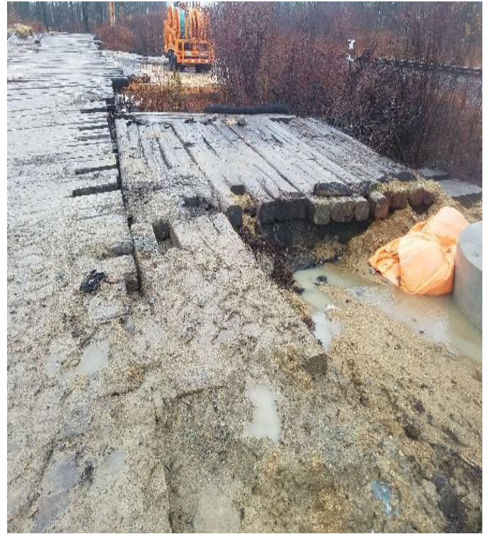
Fig 22: Turbid water from stockpiled soil flowing under mats around Str. 2. Viewing north. (12-14-19).
