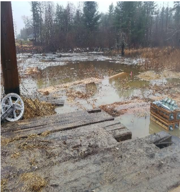
Fig 23: Area around Str. 3. No BMPs installed between work pads and wetland MW2. Viewing south. (12-14-19).
