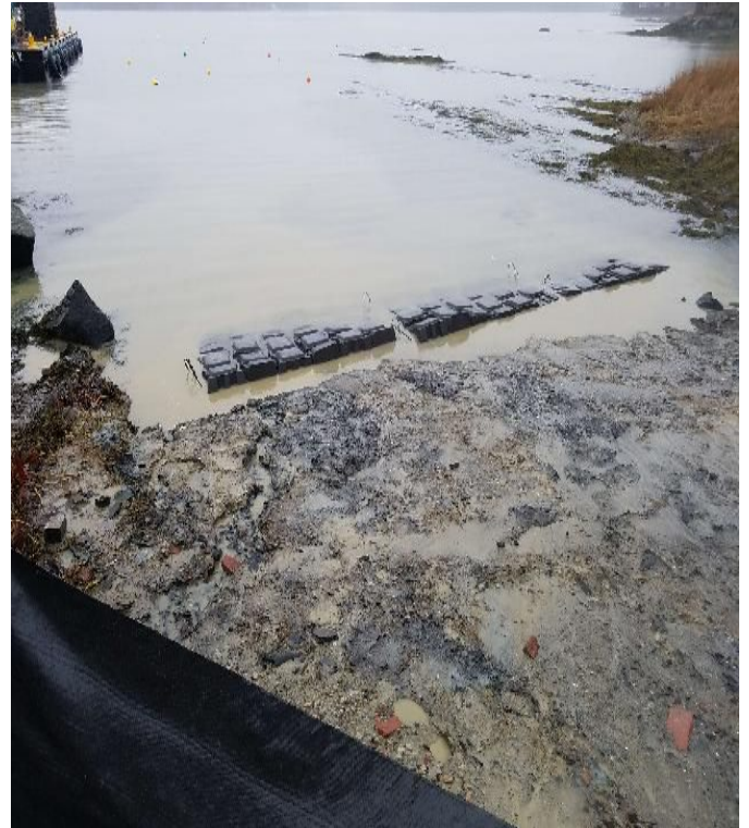
Fig 14: Concrete mattresses installed at Getchell property/west side of the Bay. Viewing wet. (12-14-19).
