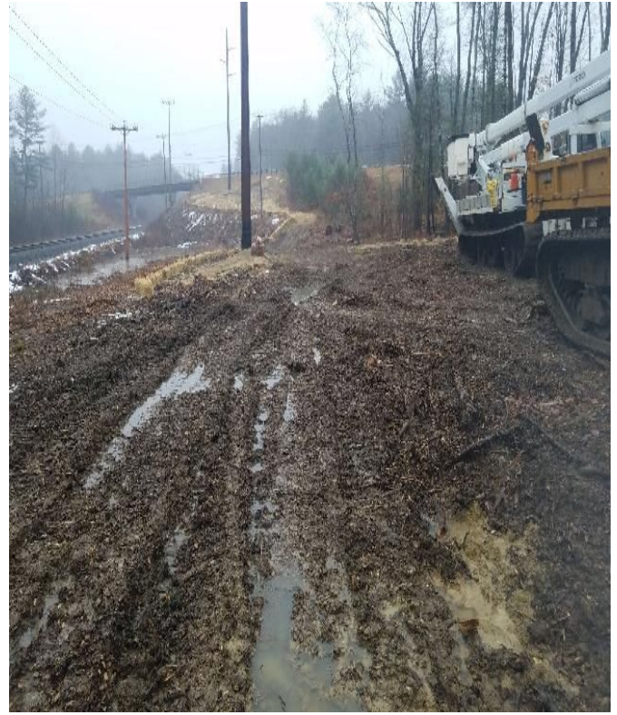
Fig 18: Ruts in access road to Strs. 5 and 6. Viewing south. (12-14-19).
